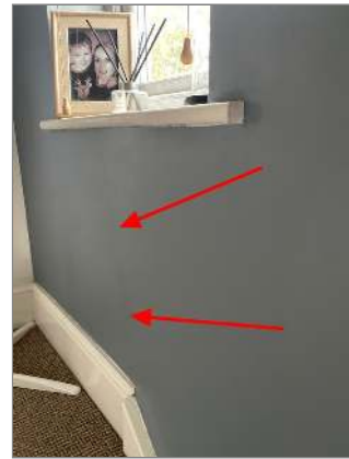
Photo - 69 Slight crack landing in line with the slight movement noted side elevation
