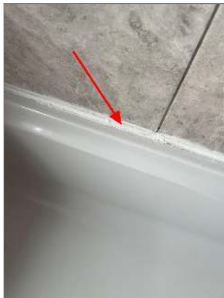
Photo - 108 Poor bath seals
