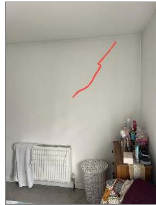
Photo - 86 Minor plaster cracks front bedroom
