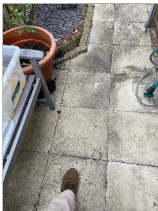
Photo - 158 Loose paving
