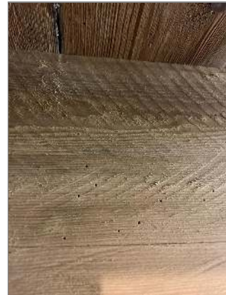
Photo - 131 Past wood worm floor yimbers seen in cellar.
